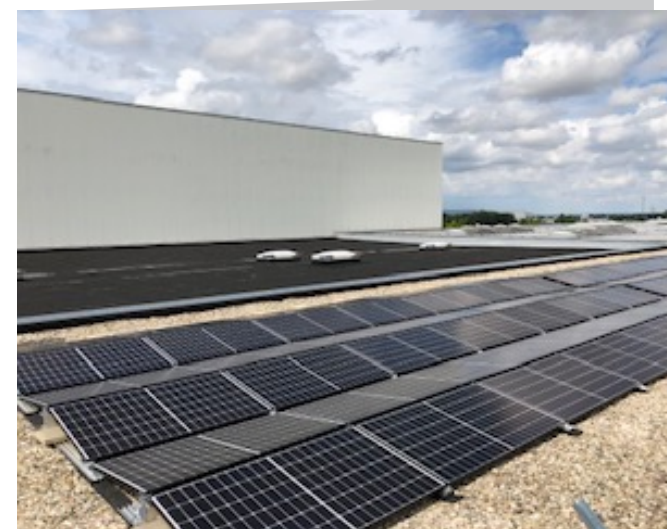
Photovoltaic facility on the roof of the new narcotics warehouse
