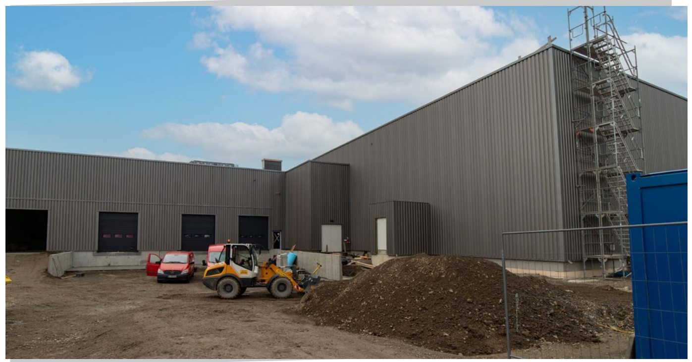
The narcotics warehouse near completion; Sustainability was given top priority during the construction process.
